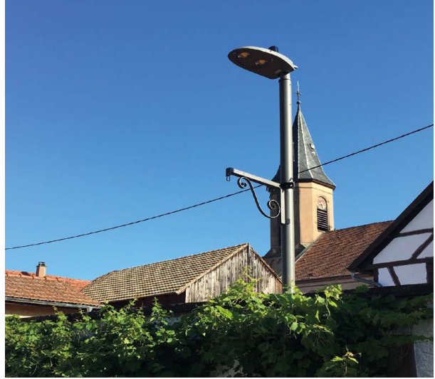
Smart Street Lighting in Alsace, France Extreme Ultra High Efficiency Series
